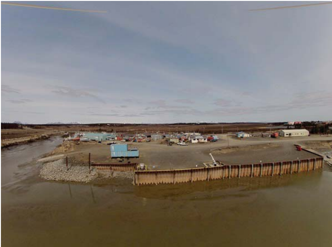
Riprap and sheetpile protection on the east side of the entrance channel, May 2014
