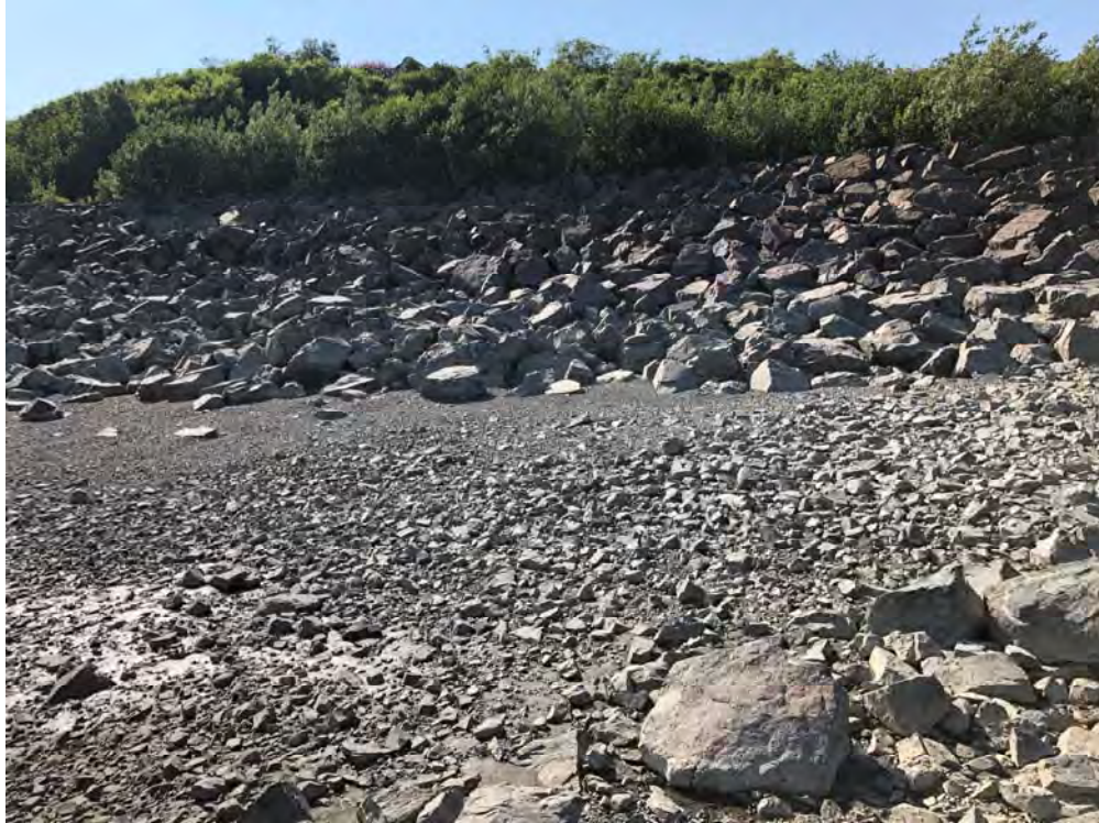
Photo 9 - Bank Armoring Between Sheetpile Wall and Outfall (Looking Northwest from Outfall at Low Tide)
